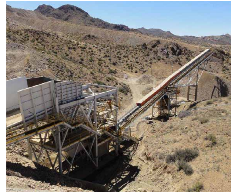
Primary crusher and live ore stockpile
