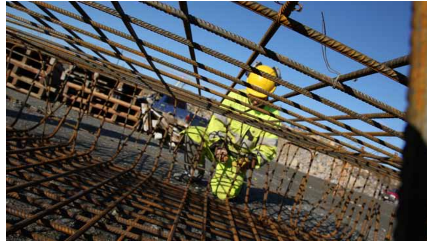
The company is in the construction phase of a uranium recovery plant
