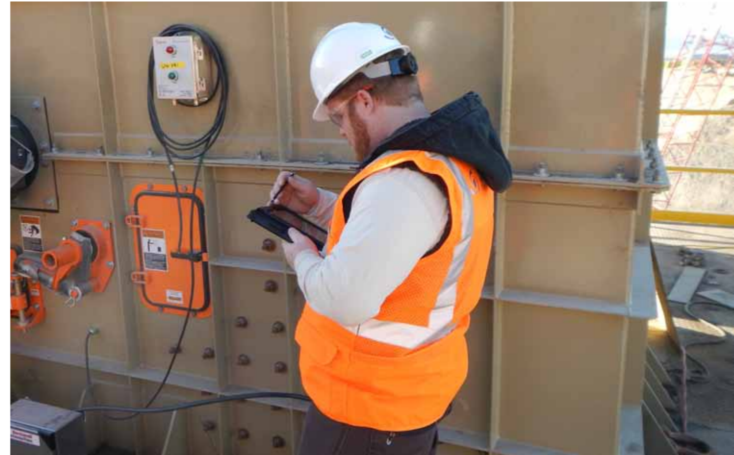
RCC engineer, Michael Toone, utilizing PlantSight while commissioning
