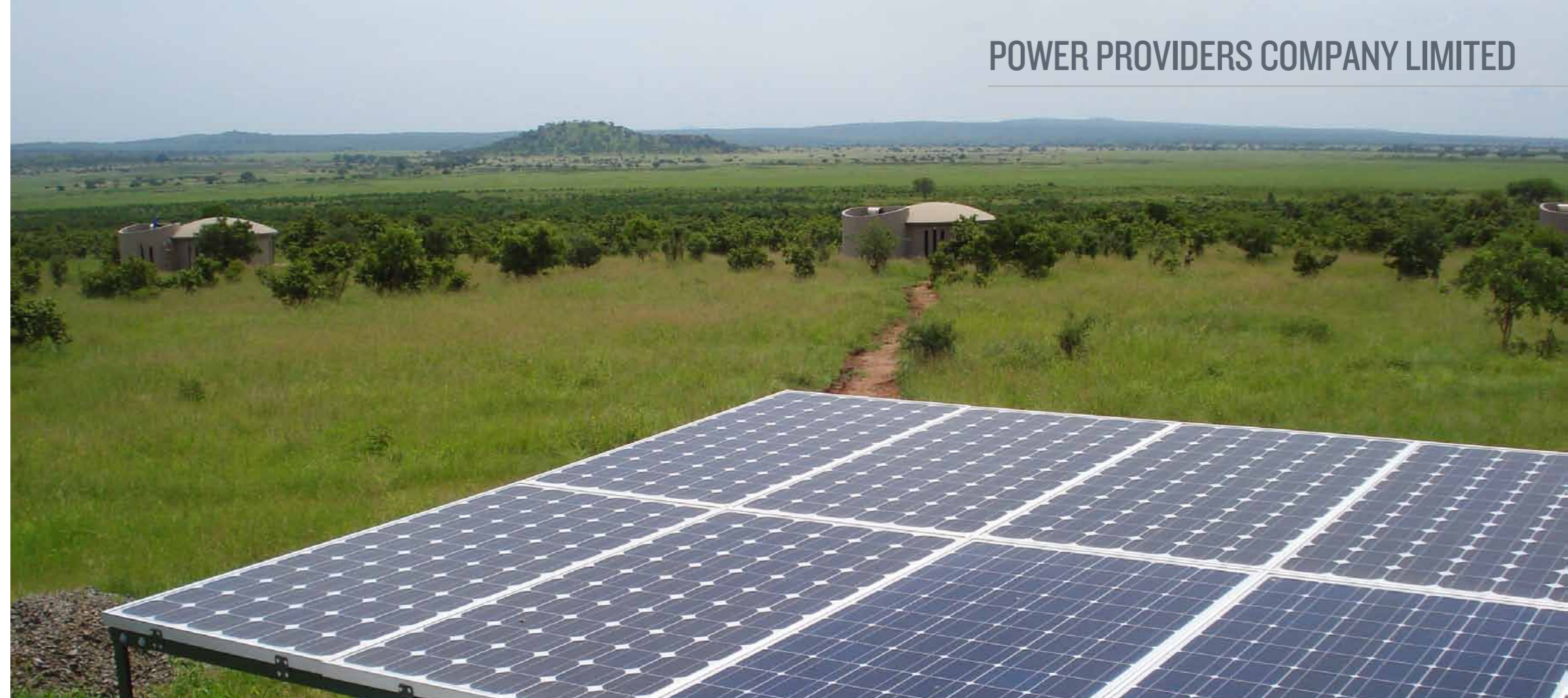
Solar array at remote bush lodge
