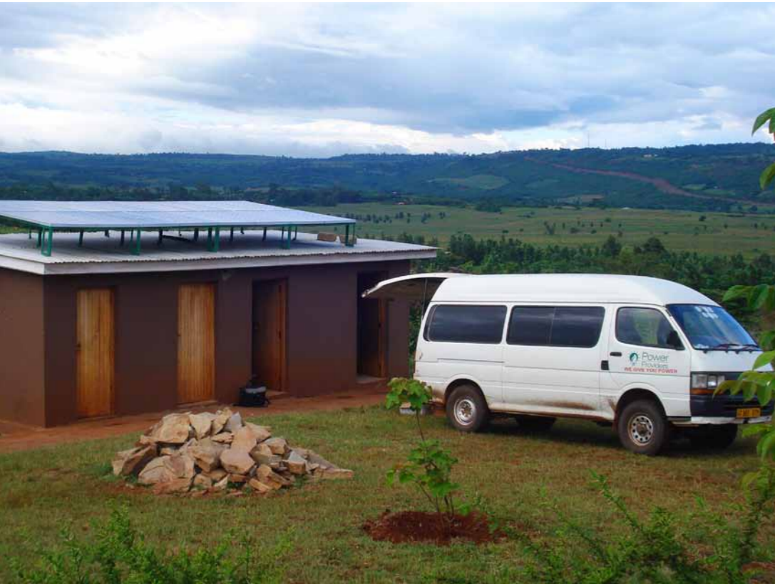
Solar array on power house
