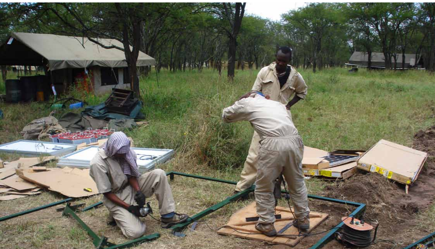
Tented camp solar installation
