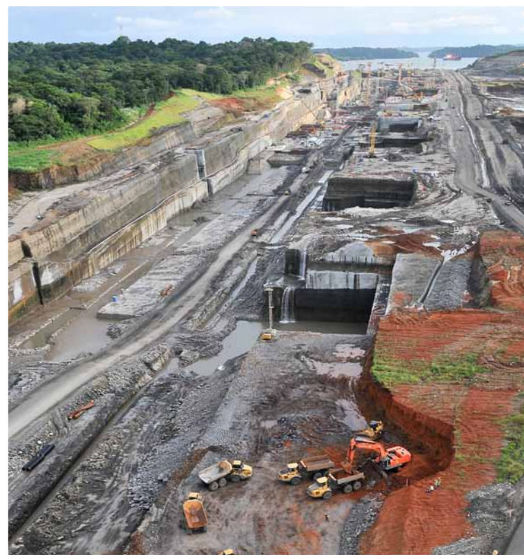
Construction and excavation of the new Atlantic Lock. In the background is Lake Gatun with ships awaiting transit through the existing Gatun locks
