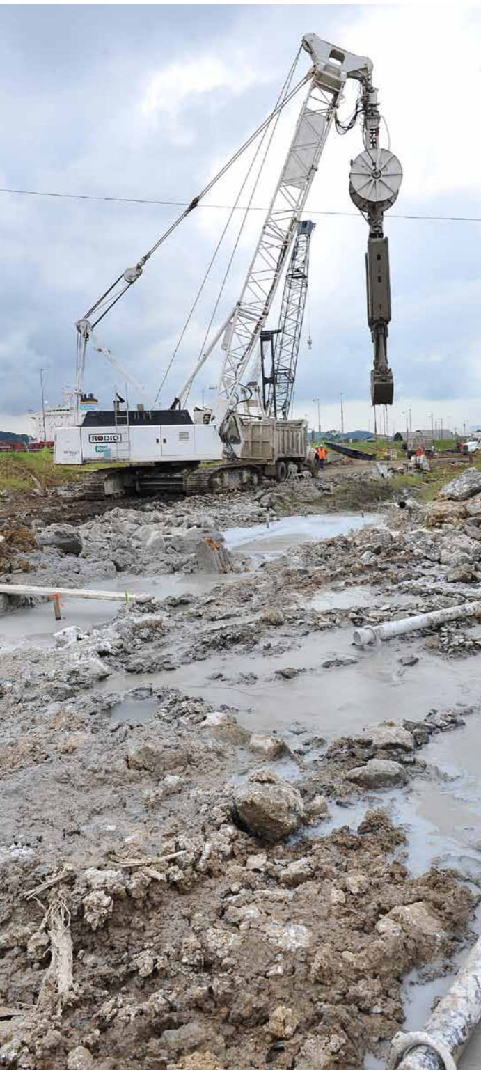
Construction of cement bentonite slurry wall between the northern end of the access channel to the new Pacific Lock and the exiting Pedro Miguel Locks
