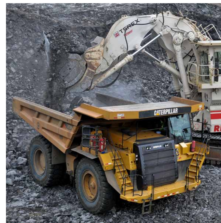
Basalt excavation of the access channel that will connect the new Pacific Lock to Gatun lake at Culebra Cut
