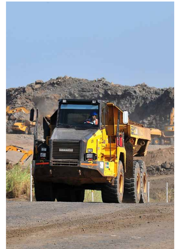
Excavation of access channel that connects the new Pacific Lock to the Culebra Cut
