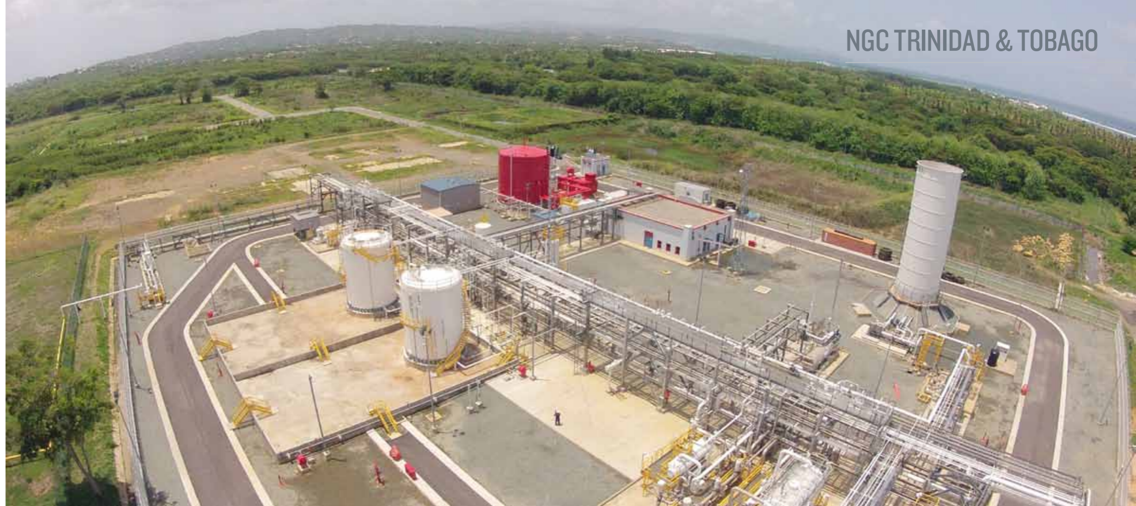
NGC Tobago pipeline gas receiving facility
