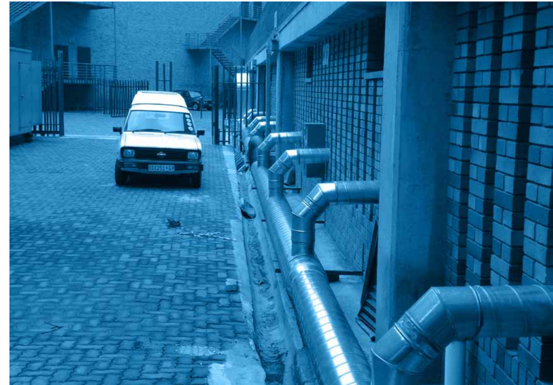
Ducting at University of Johannesburg
