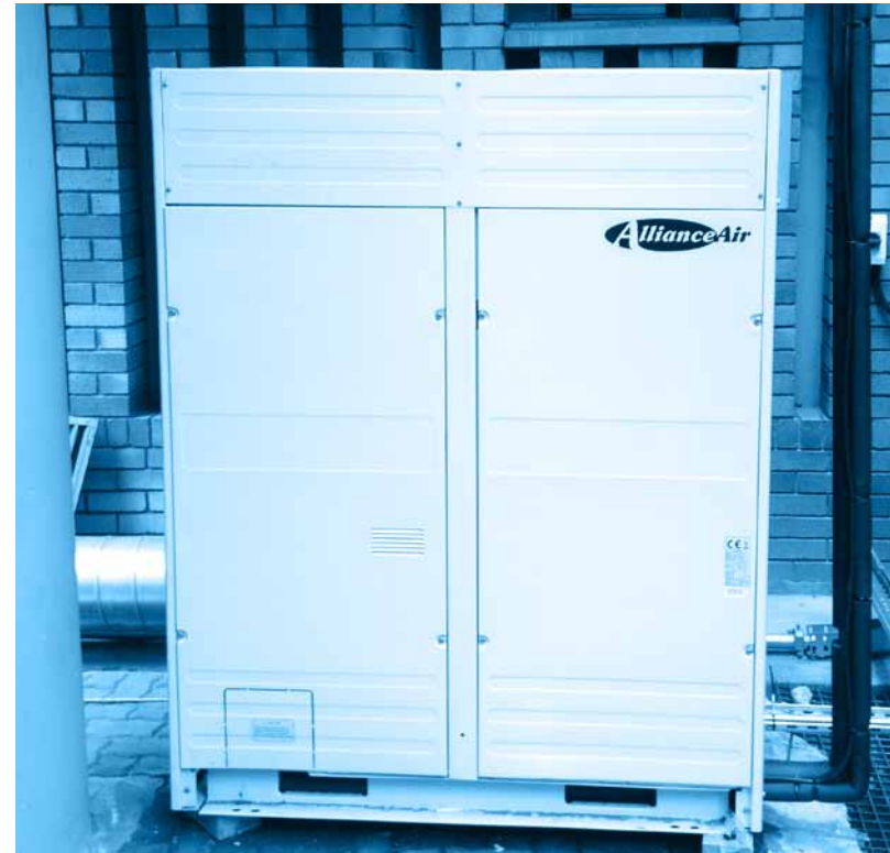
Installed unit at University of Johannesburg
