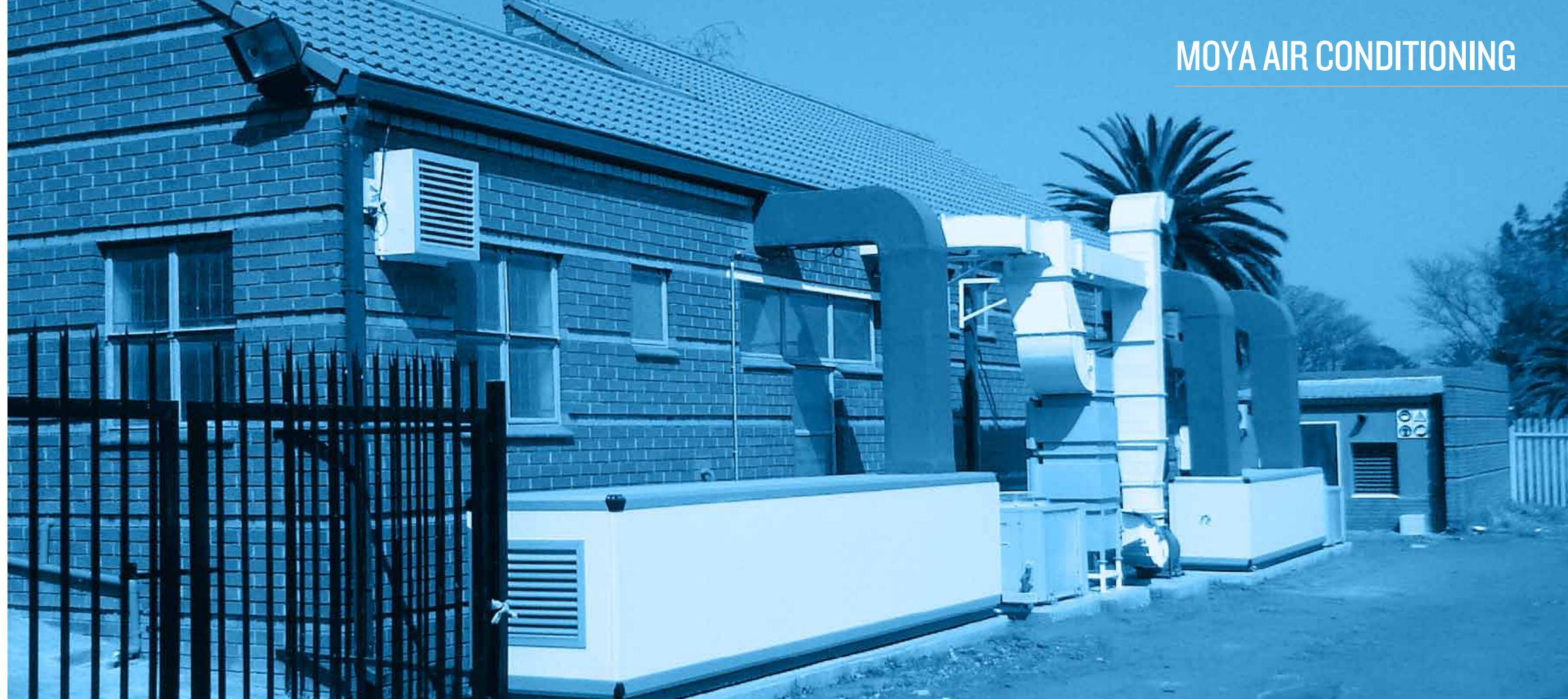
South African National Blood Service air handling units, clean room
