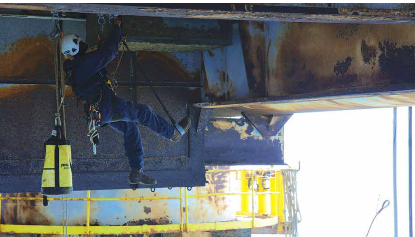
Working from ropes is the access method of choice for inspection work
