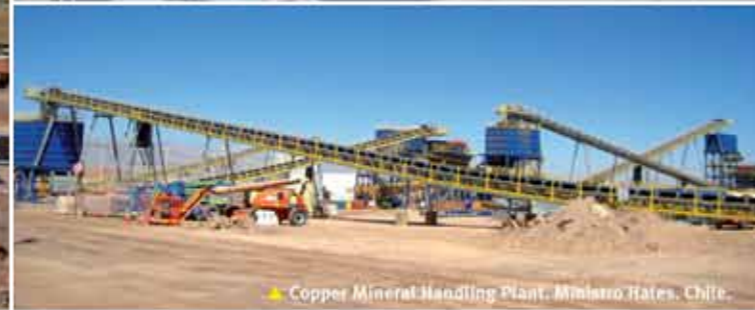
▲ Copper Mineral Handling Plant, Ministro Hates, Chile.
