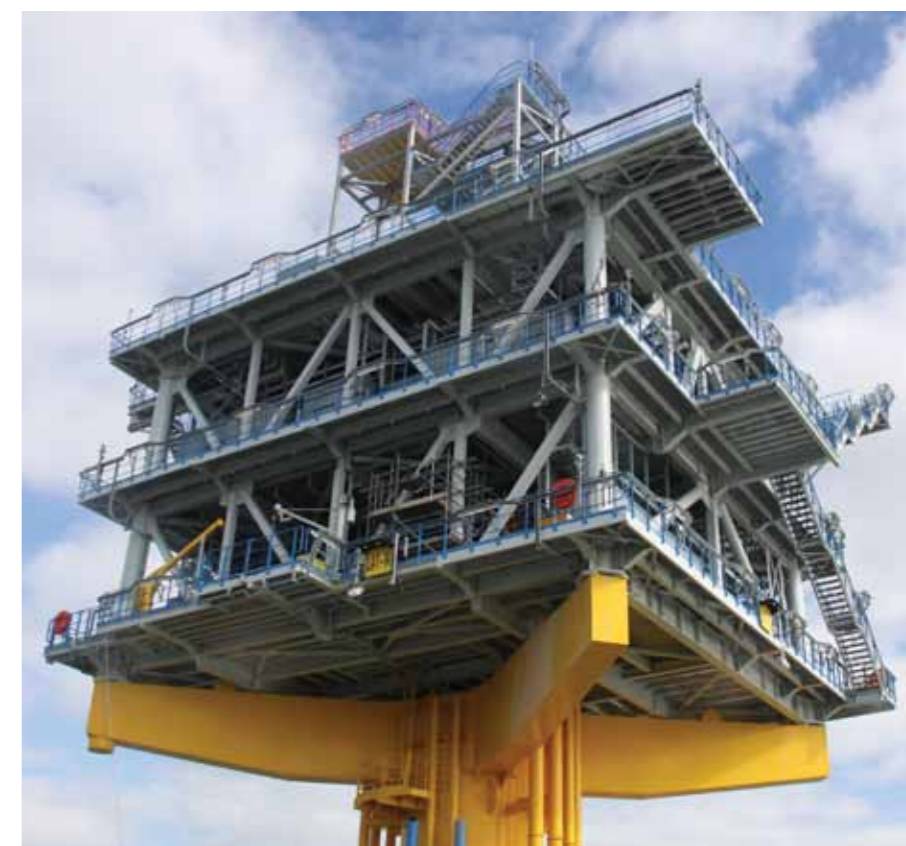
Offshore substations boost the voltage to reduce transmission losses
