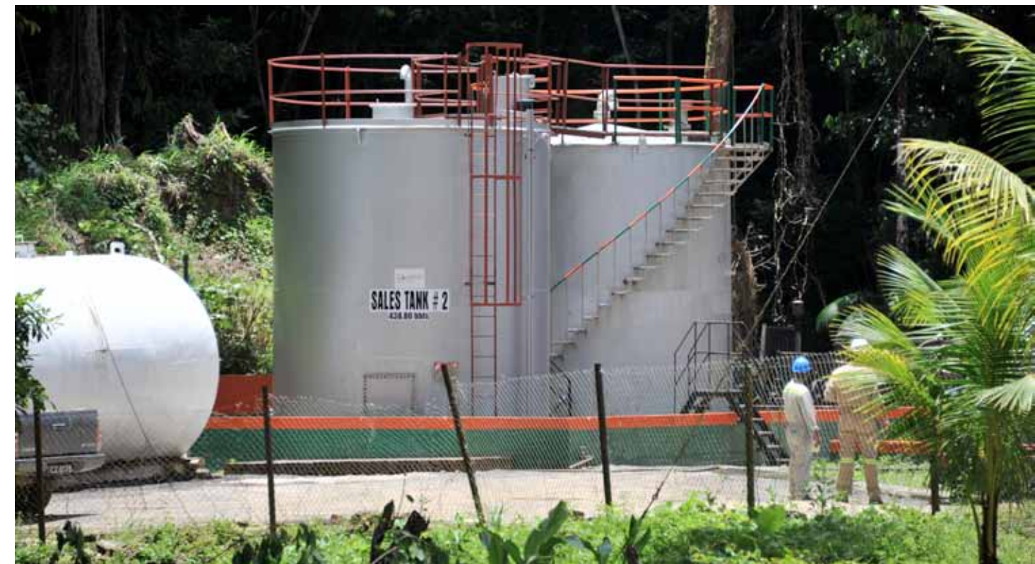
Sales Tanks 1 and 2 at Goudron
