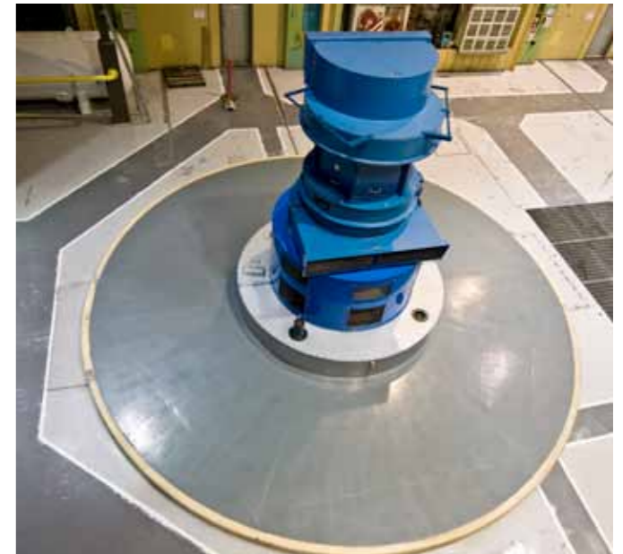
Water turbine generator
