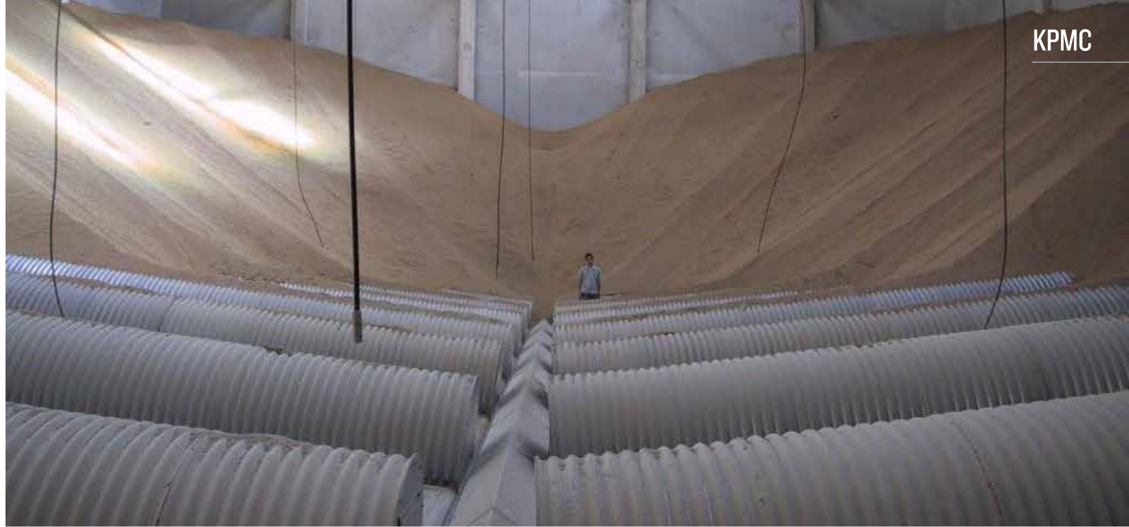
Vibrating floor clearing a grain silo
