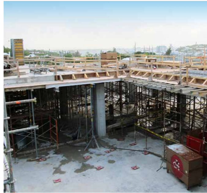
The new hospital facility under construction, looking down the atrium from the third to the second floor
