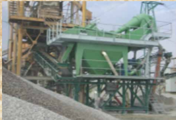
SAND TREATMENT UNIT
