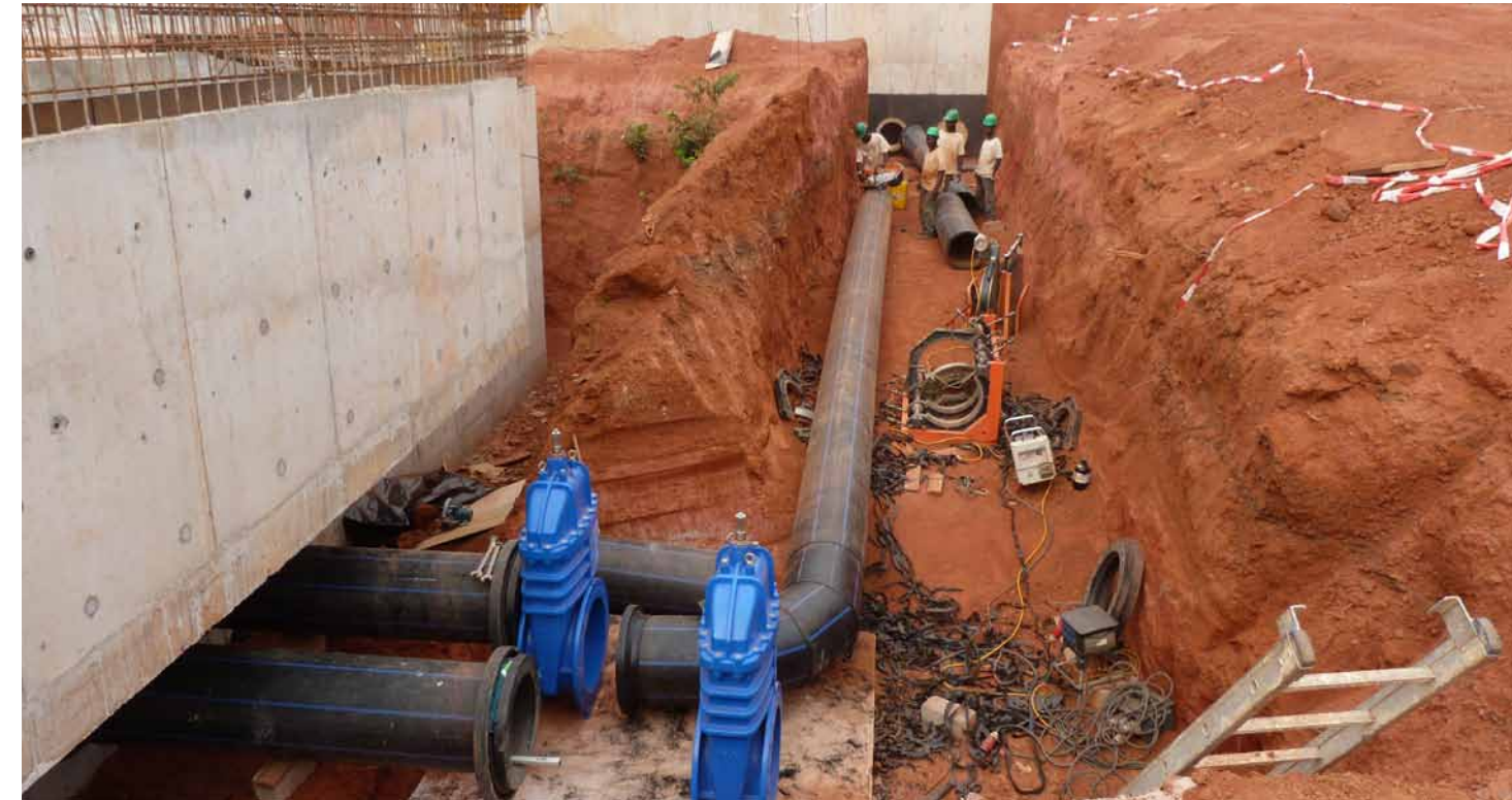
Pipe interconnection to treatment plant at Essakyir
