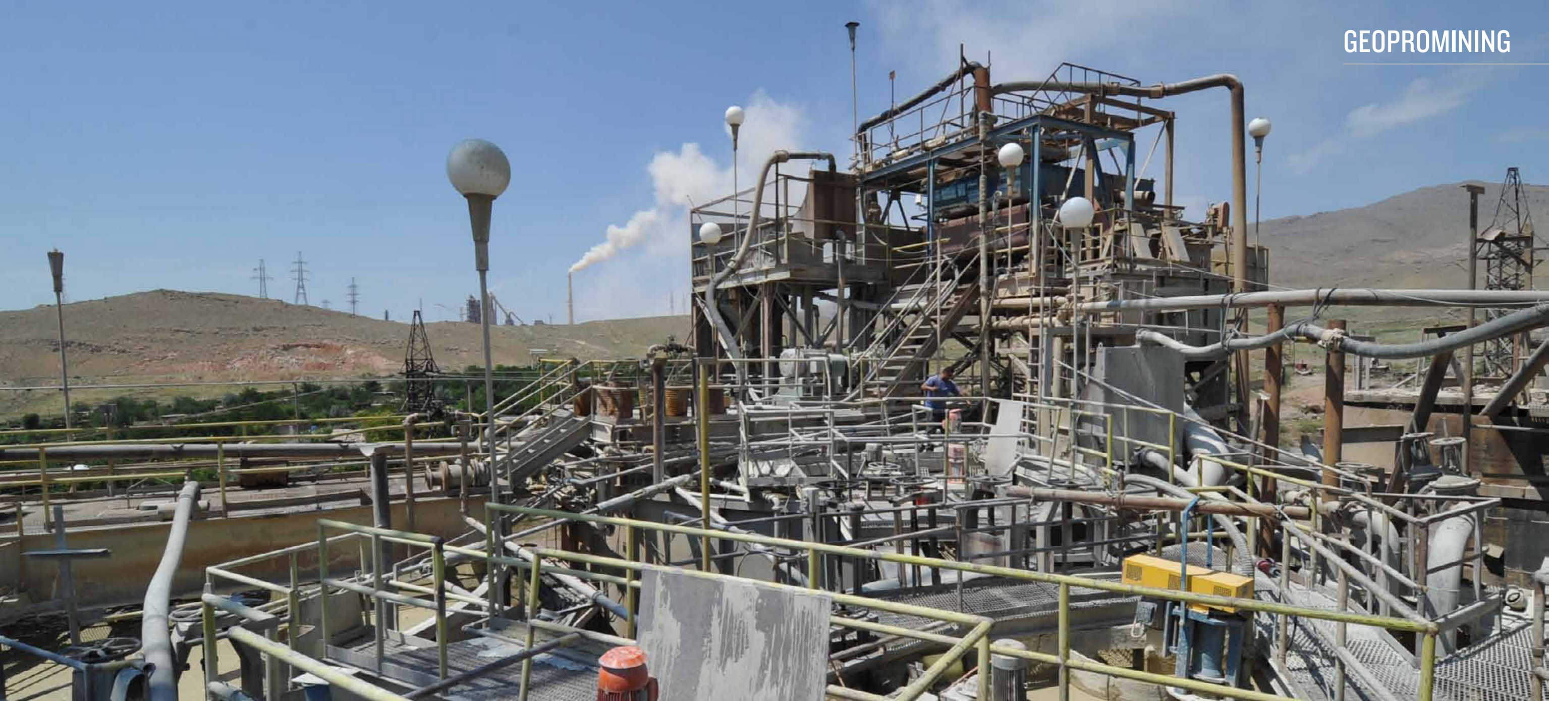
Leaching tanks at the Ararat gold recovery plant in Armenia
