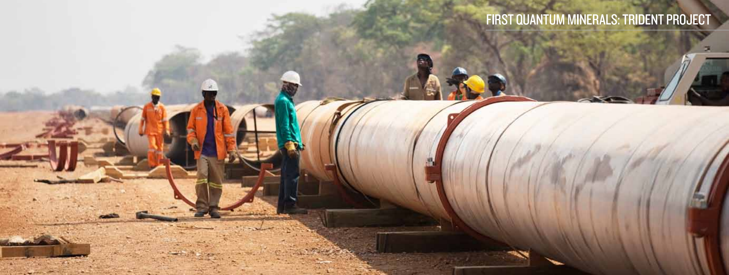
The 14km pipeline to the Chisola Dam will supply process water to the plant
