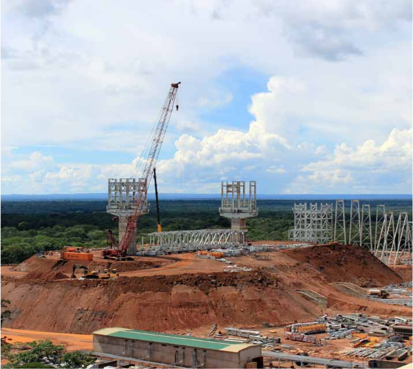
The crushed ore stockpile at Sentinel has 80,000 tonnes of live capacity and is roughly the size of Lusaka football stadium
