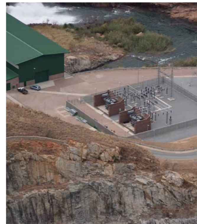
Maguga substation, Swaziland
