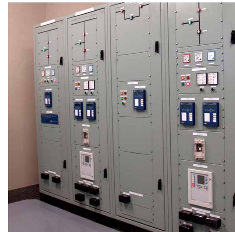
Control panels, Eastgate substation
