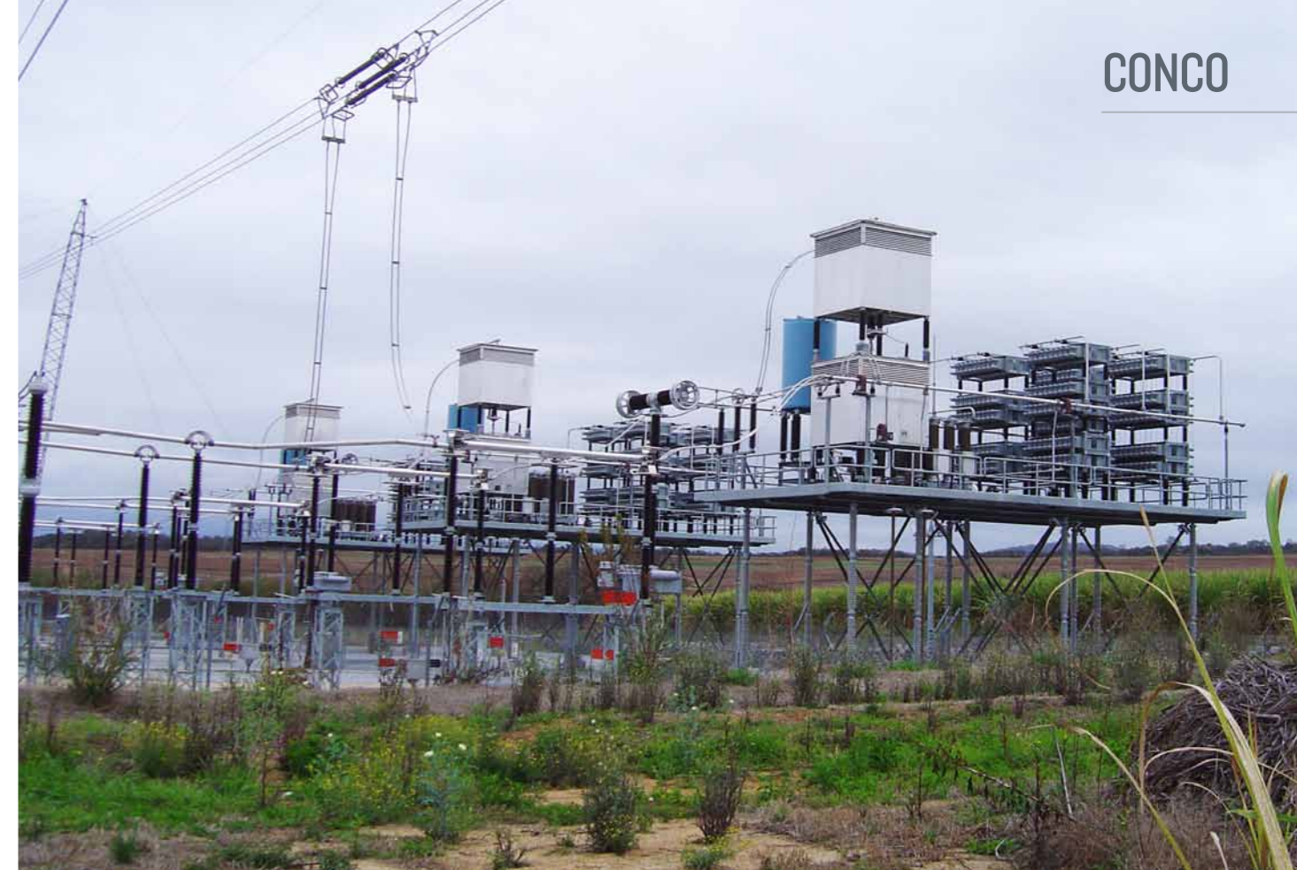
Motraco substation, Mozambique
