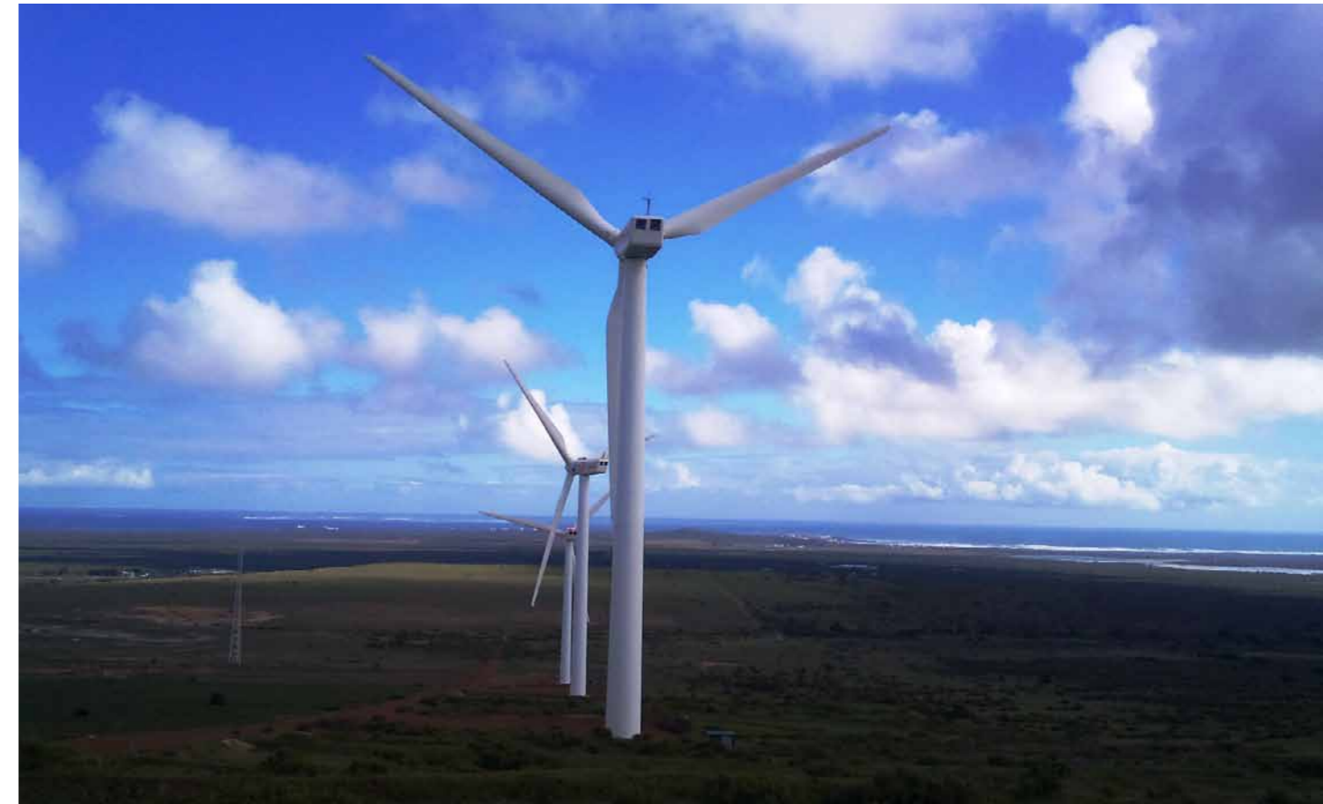
Darling wind farm
