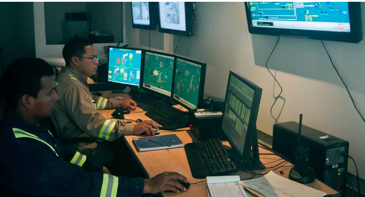
Control room to monitor the process of Petaquilla Gold LTD
