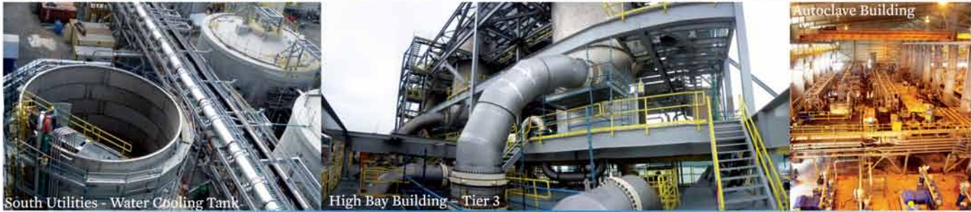
South Utilities - Water Cooling Tank
