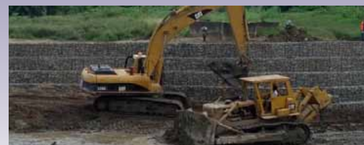
INDRHI AND INTERNATIONAL WORLD BANK IRRIGATION PROJECTS Lote 10, Jima Camu siphon and irrigation pumping system, La Vega, Dominican Republic.
