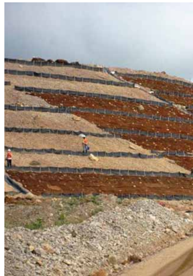
Coconut mats are laid along the slopes of a recently-constructed access road to aid in soil stabilisation
