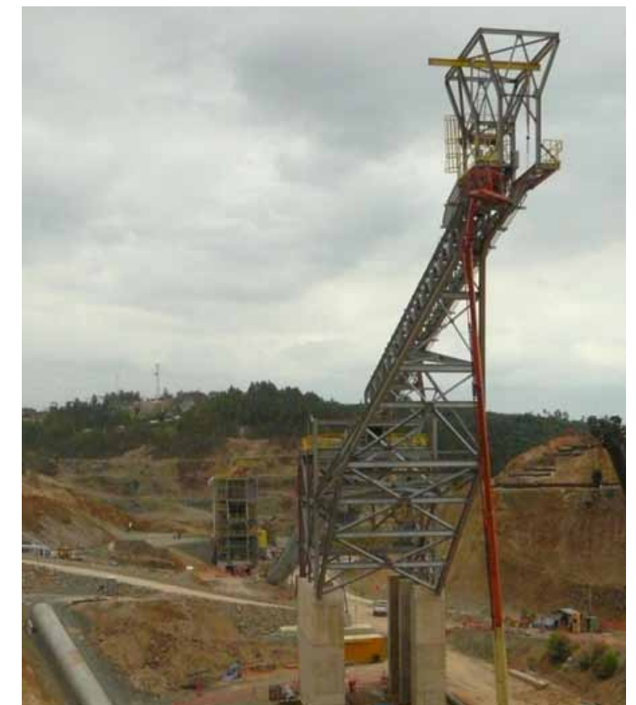
Construction in progress on the primary ore crusher, ore stacker foundation, and ore reclaim feeder chamber
