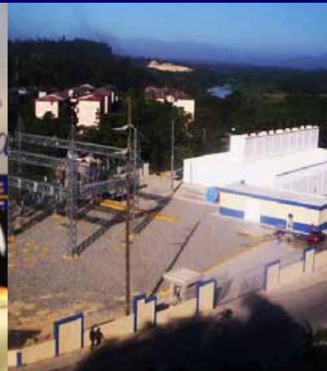
METRO SANTO DOMINGO line I y II, Emergency Power Generation plant, 40MVA and Substation 138KV/40MW.
