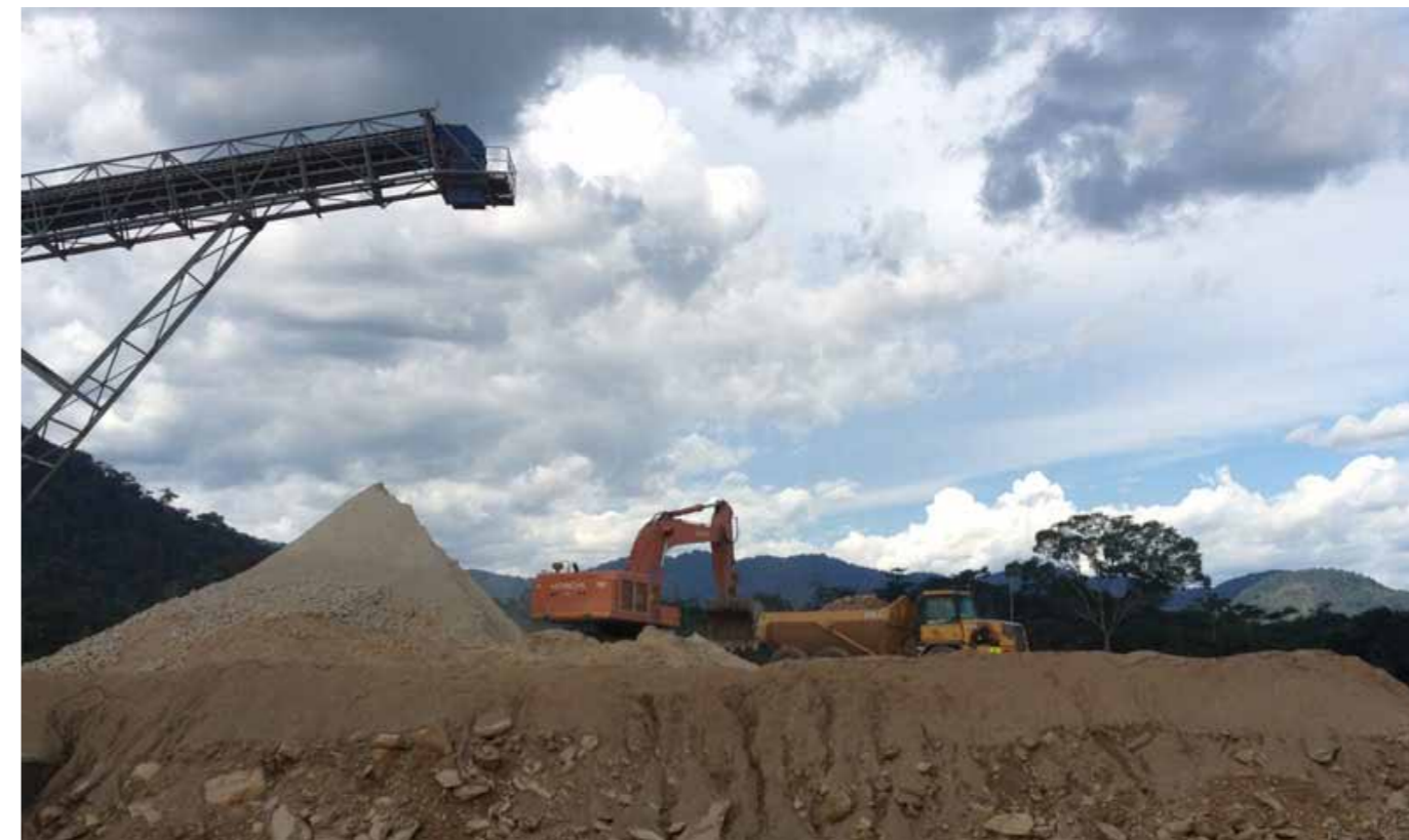
Re-handling of crushed ore from the primary product stockpile to the heap leach pad
