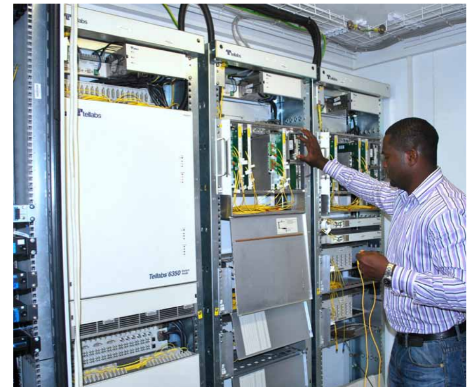
Telecom engineer testing the signal to identify the loss of signal location along the fibre optic route
