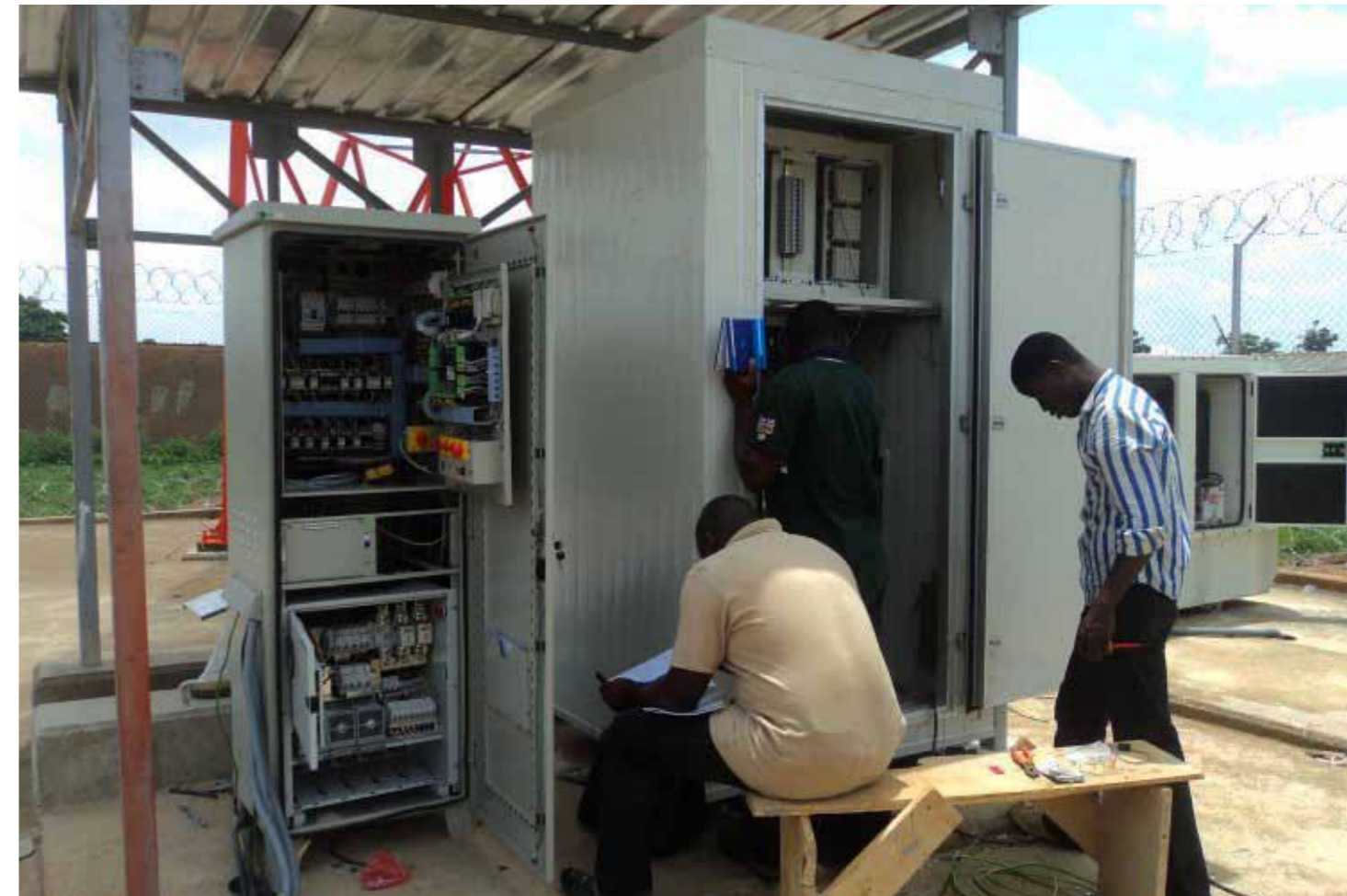
Installation of a hybrid controller on BTS site which reduces the diesel consumption of the generators
