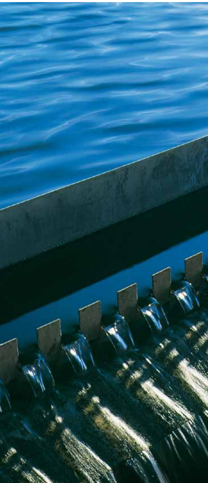
Detail of one the installations at La Farfana sewage treatment works in Chile
