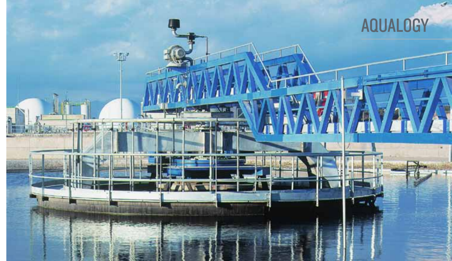
One of the installations of La Farfana sewage treatment works in Chile
