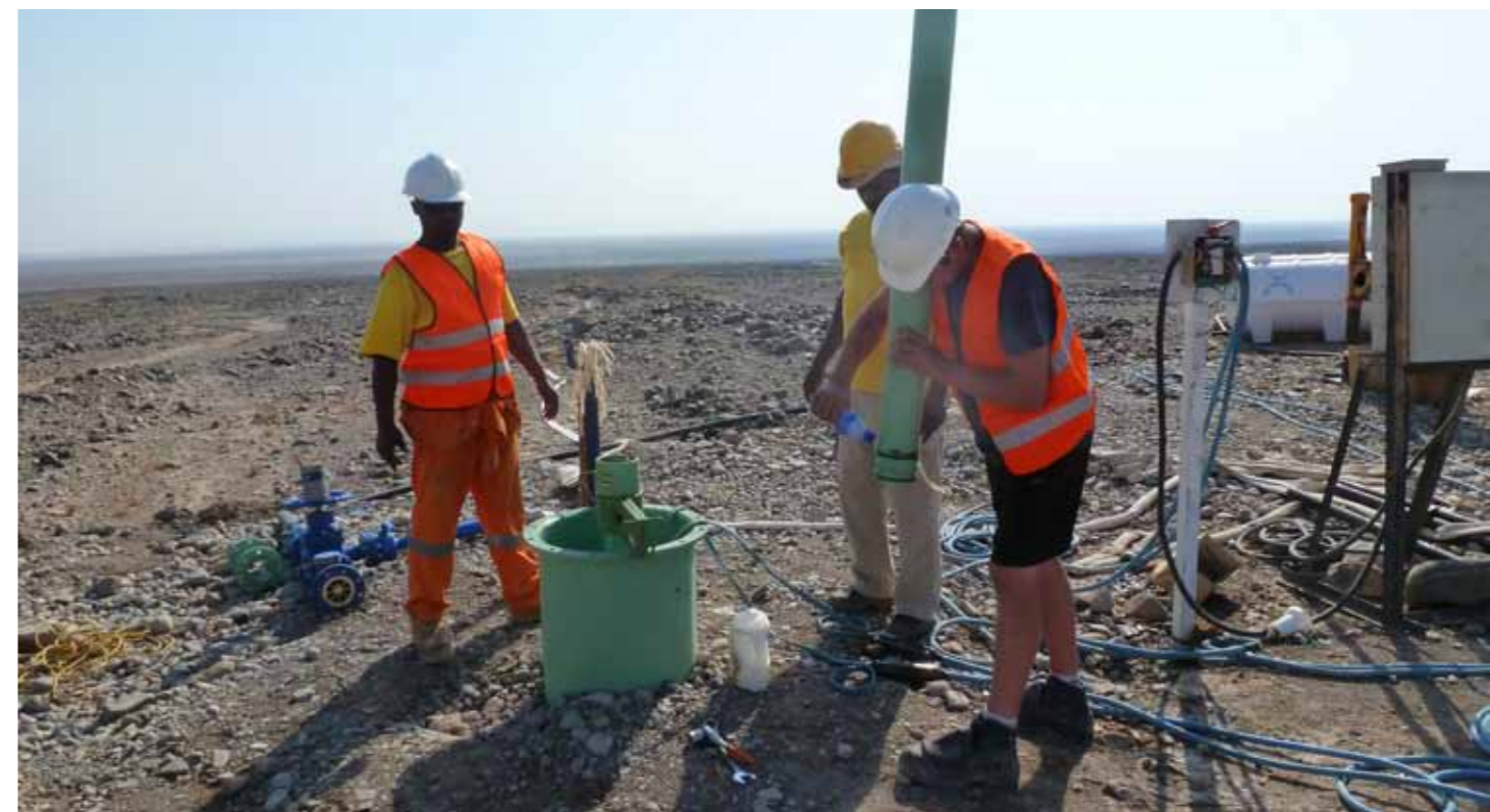
Production water well wellhead assembly
