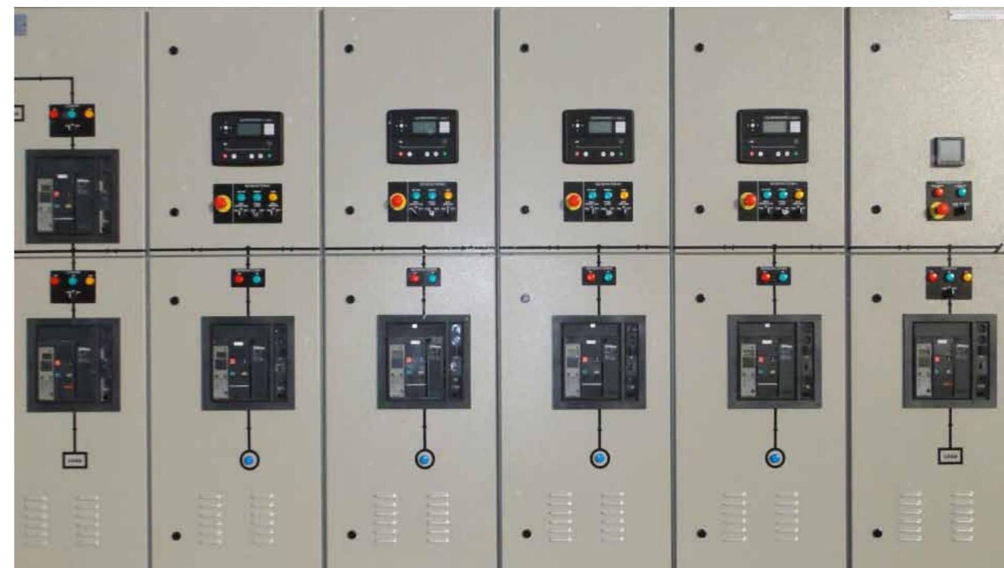
Generator sync panel
