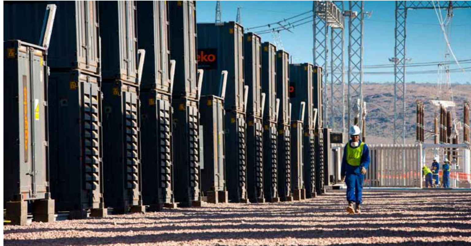
Aggreko power plant, Ressano Garcia, Mozambique
