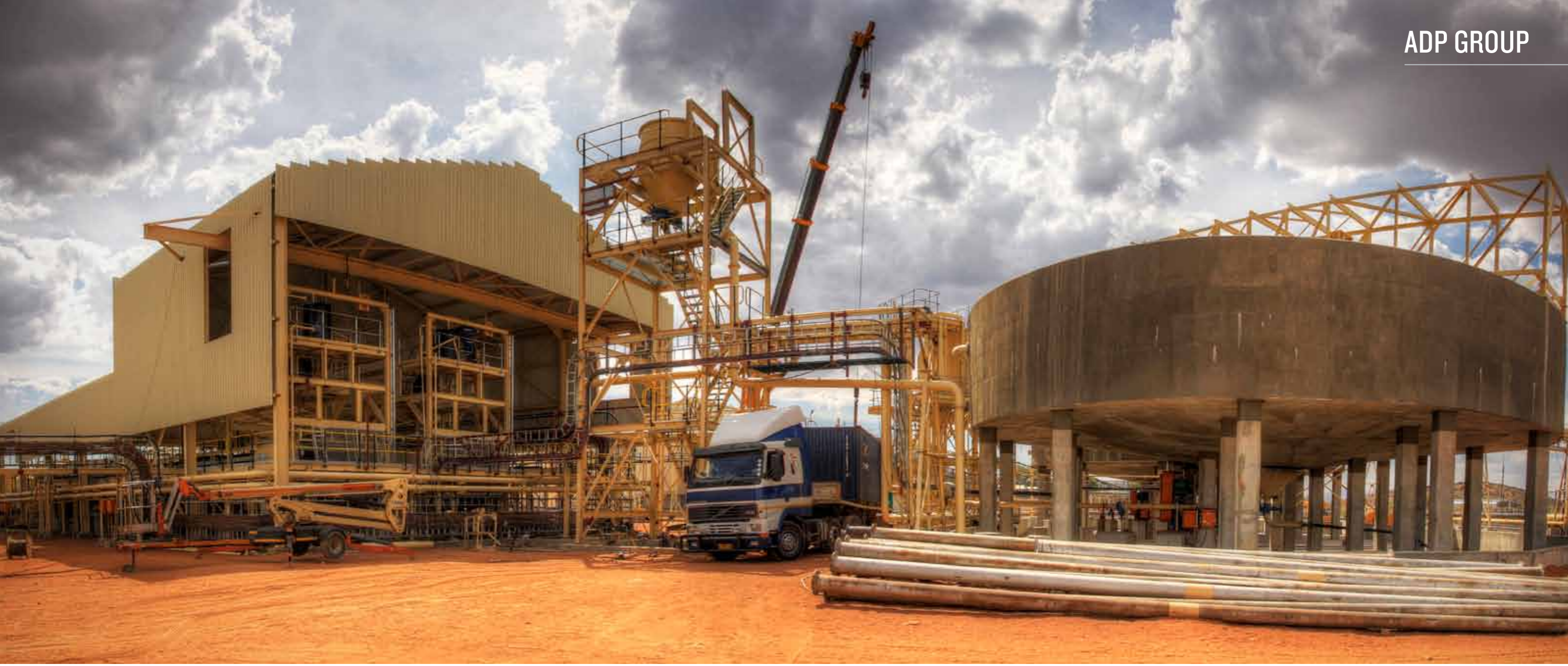
Navachab filter plant and thickener
